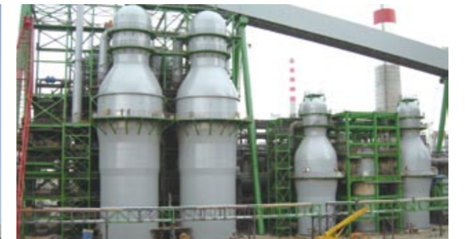
首钢京唐2号高炉热风炉 Hot blast stoves for Shougang Jingtang 2# blast furnace
