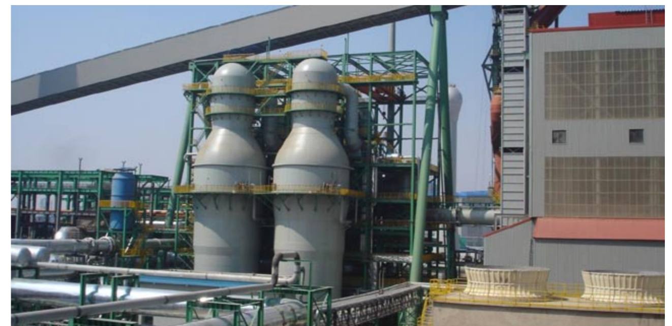
首钢京唐5500m³高炉的4座热风炉采用非对称矩形布置 Asymmetric rectangular arrangement of 4 hot blast stoves used for Shougang's Jingtang 5500m³ blast furnace
