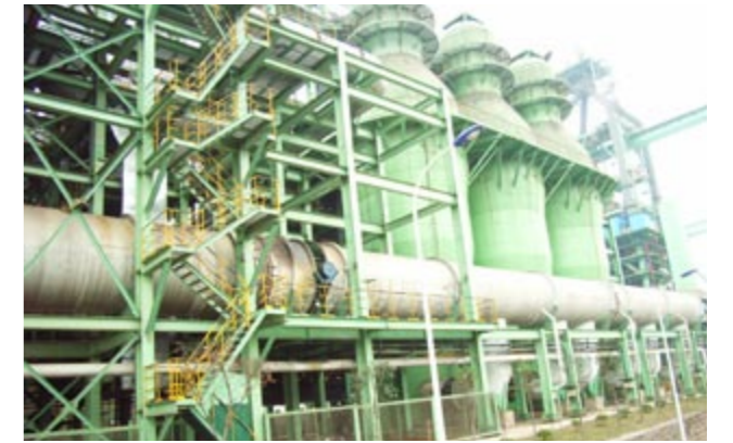
重钢4号高炉热风炉 Hot blast stoves for Chonggang 4# blast furnace
