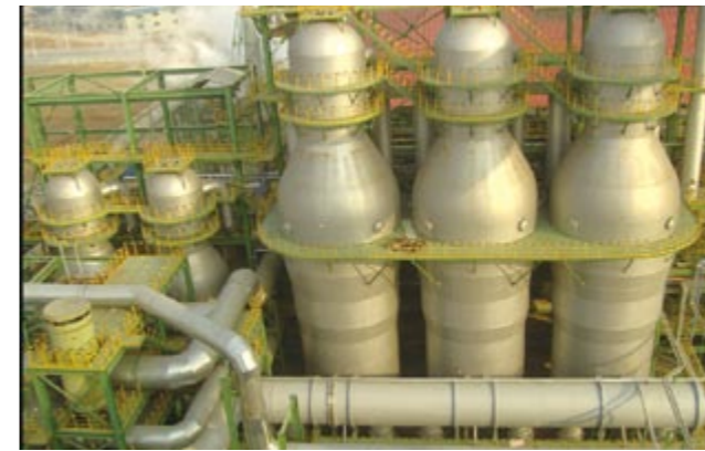
首秦1号高炉热风炉 Hot blast stoves for Shouqin 1# blast furnace
