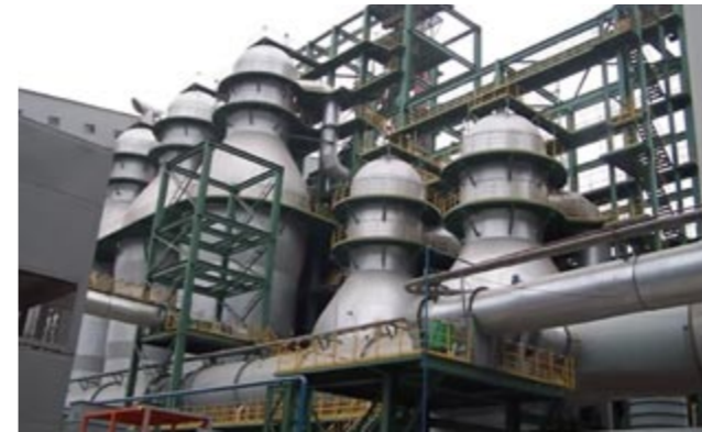
首秦2号高炉热风炉 Hot blast stoves for Shouqin 2# blast furnace
