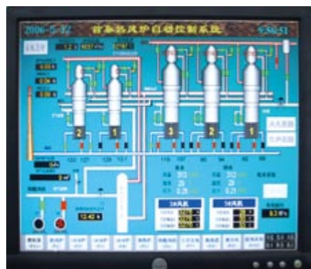
助燃空气高温预热控制画面 Control image of high-temperature preheating of combustion air
